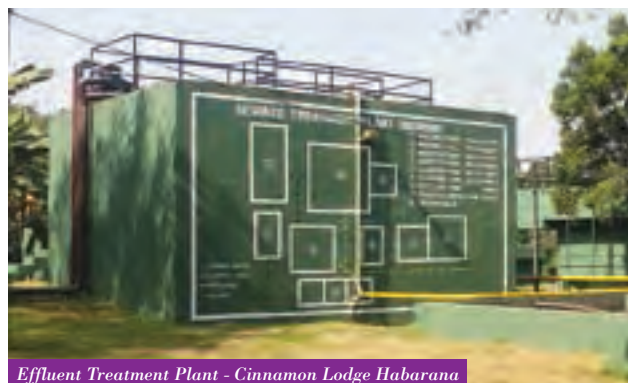
Effluent Treatment Plant - Cinnamon Lodge Habarana
