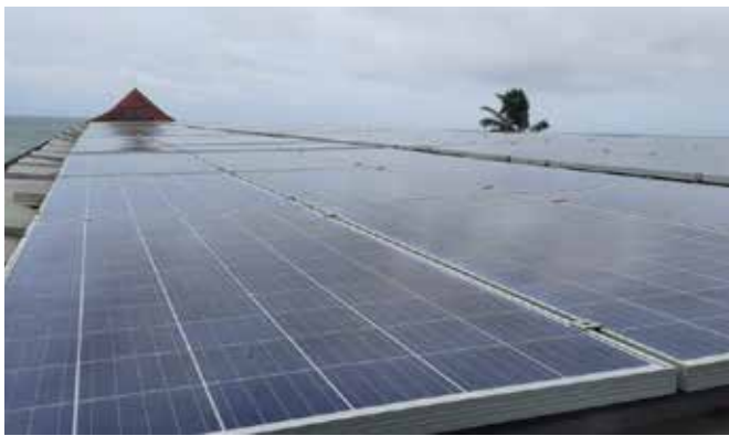
Solar PV System - Hikka Tranz by Cinnamon
