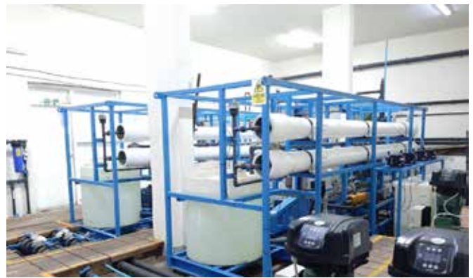
Water Treatment Plant - Cinnamon Velifushi Maldives
